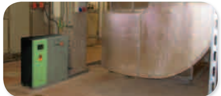
humiFog in equipment room
